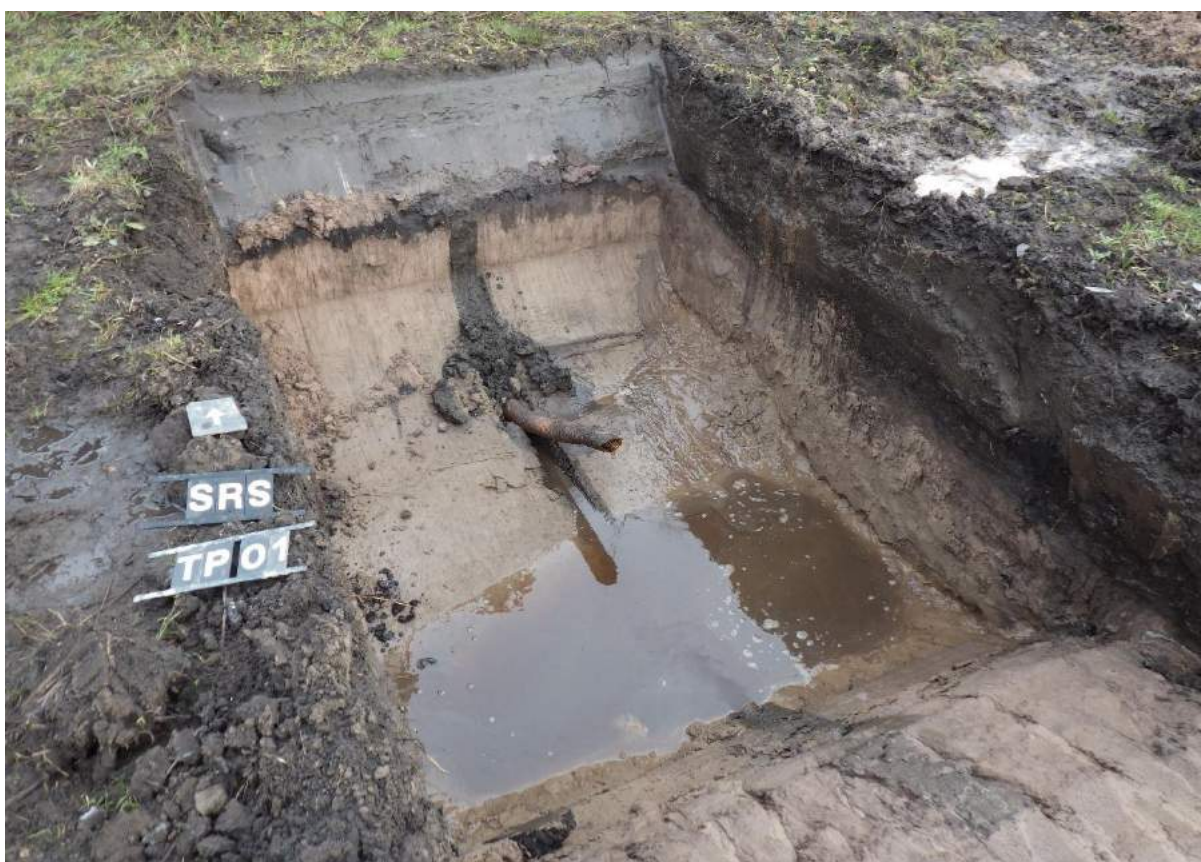
Plate 18: Test Pit 1 (TP01) carried out at the northern end of Trench 1. Test Pit terminated at 1.10m BGL due to pipe struck, previously obscured by groundwater ingress
