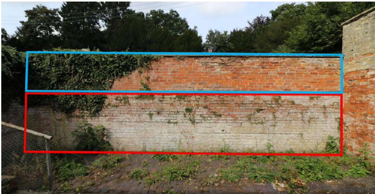
Figure 49 The north wall of the wash yard. 18 th century fabric marked in red and 20 th century fabric marked in blue.
