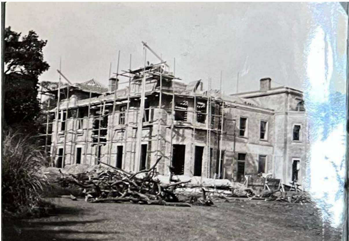
Figure 26: Photograph taken during the 1930s works to the house showing the rebuilding of the west wing after the previous wing's demolition, seen on Site visit on 22/09/22
