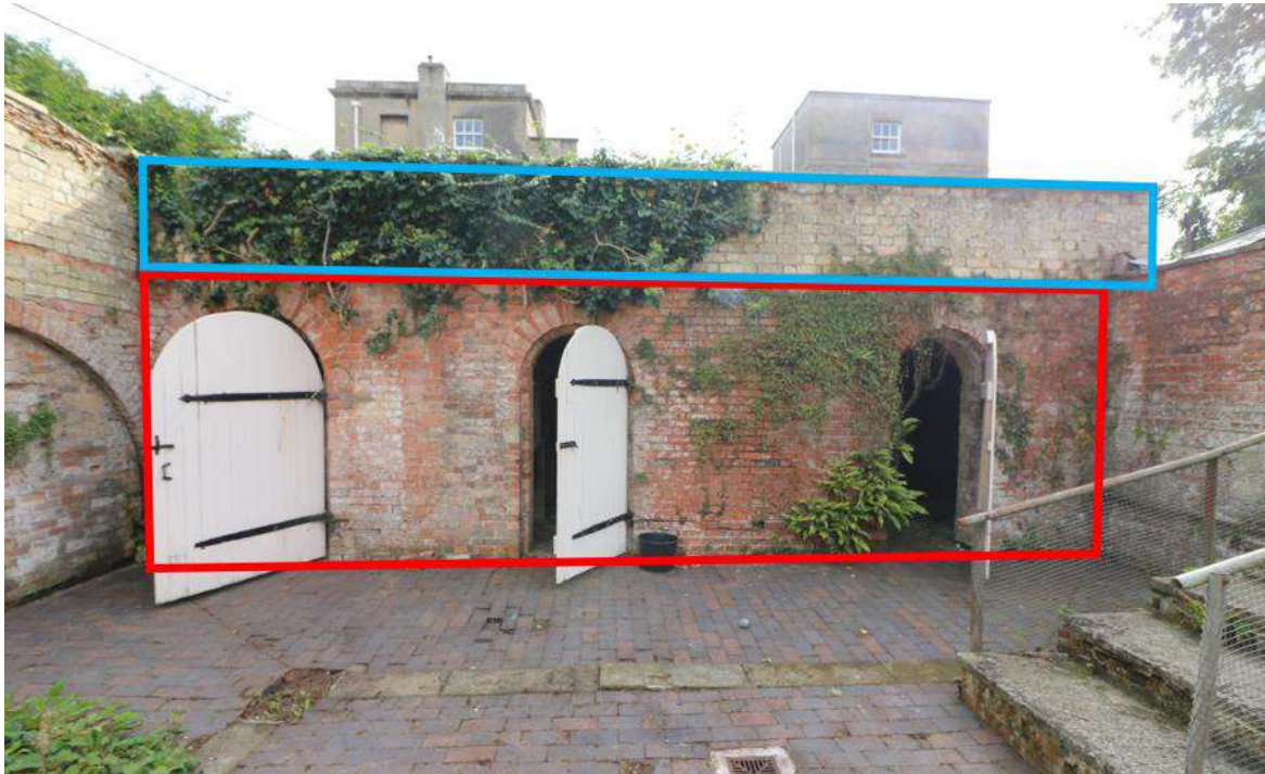
Figure 47 The south wall of the wash yard. The 18 th century phase is marked in red and the 20 th century brick parapet marked in blue.
