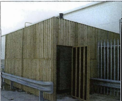
3m high enclosure for a generator
