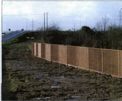
2m high barrier
