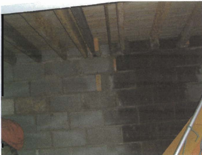
Plate 15 Damp staining in the rear wall of Room 3.
