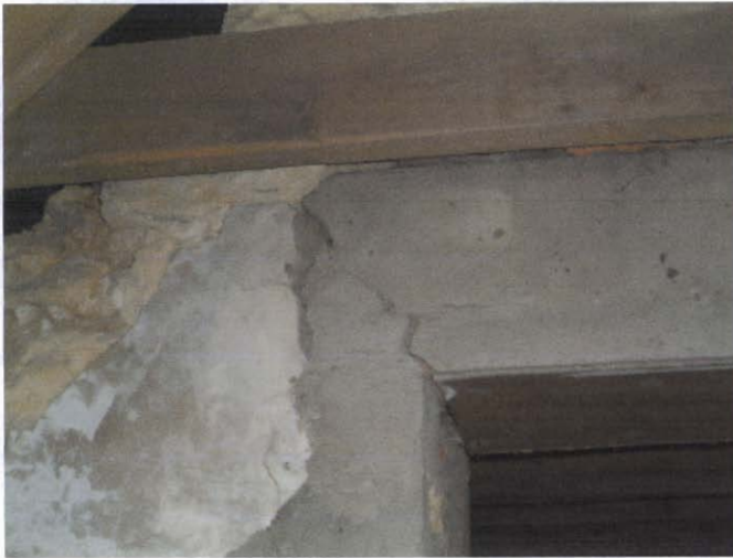
Plate 7 Cracking above the door reveal between the first floor rooms (through previous repairs).
