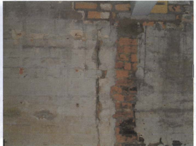
Plate 16 Vertical crack in the west (internal) wall of Room 4.
