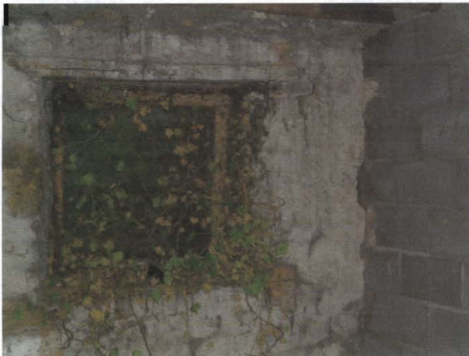
Plate 17 Growth of vegetation through the window of Room 4 (East Wall)
