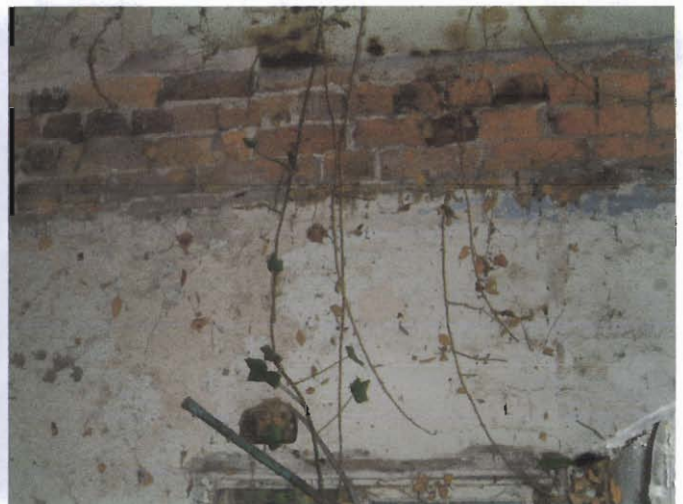
Plate 12 Vegetation inundating the openings on the western gable.
