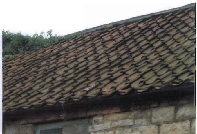
Plate 6 Undulation/distortion in the roof tiles.
