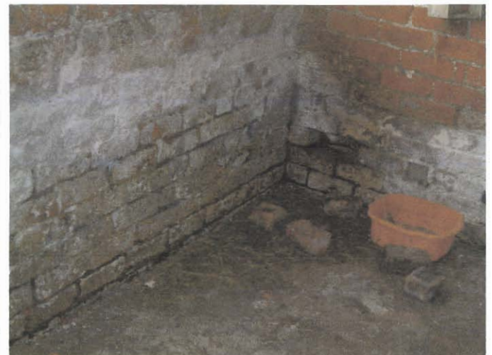
Plate 16 Low level dampness within Building 3
