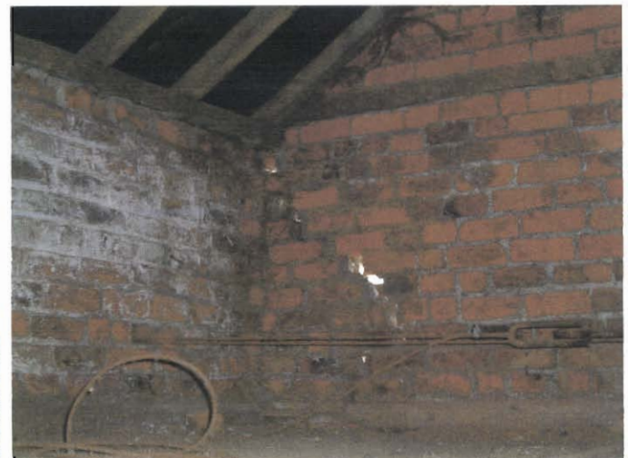
Plate 4 Substantial cracking on the east wall (internal view).
