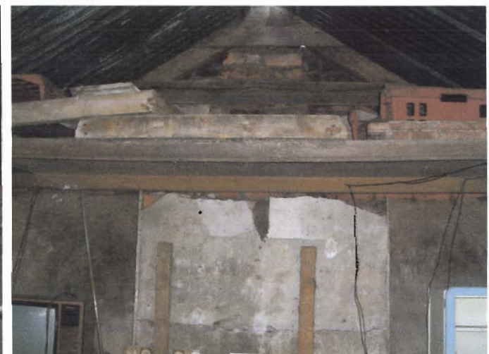
Plate 12 Roof construction over the east wall of the derelict living accommodation (Building 2).
