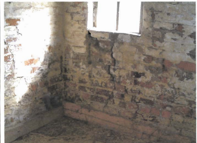
Plate 6 Cracking at ground floor level on the east gable of the barn.
