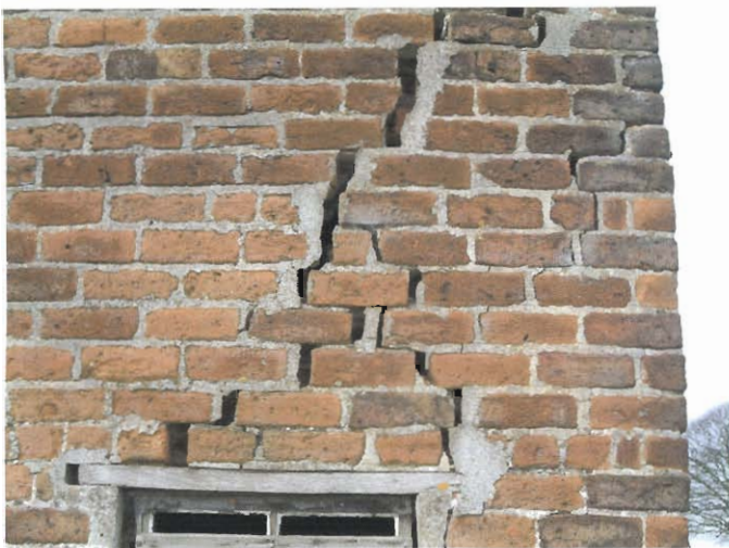
Plate 3 Substantial cracking on the east wall (external view).
