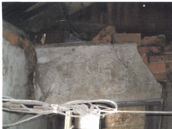
Plate 11 Partially collapsed brickwork panel over the door to the derelict living accommodation (Building 2).
