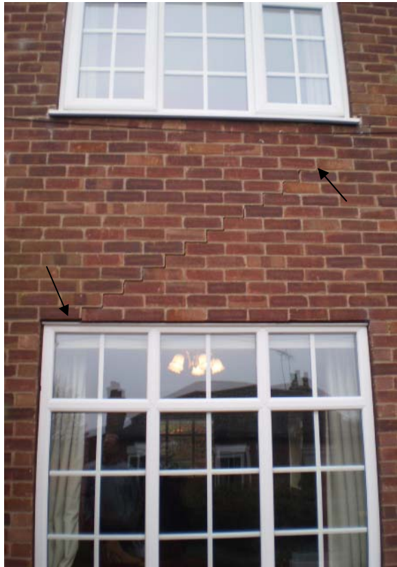
Extension right flank above ground floor window
