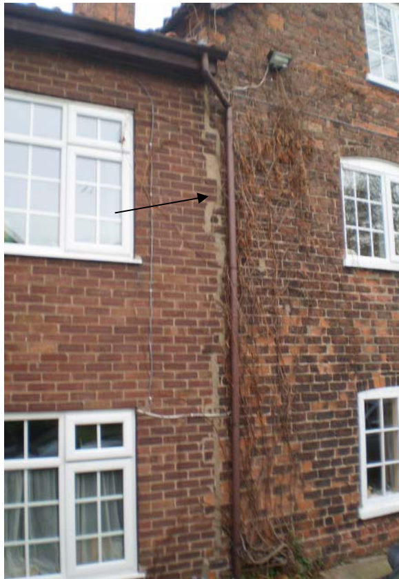
Historic damage noted to left hand flank junction of extension and main house
