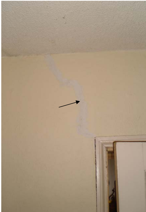
Historic damage to first floor front right hand bedroom
