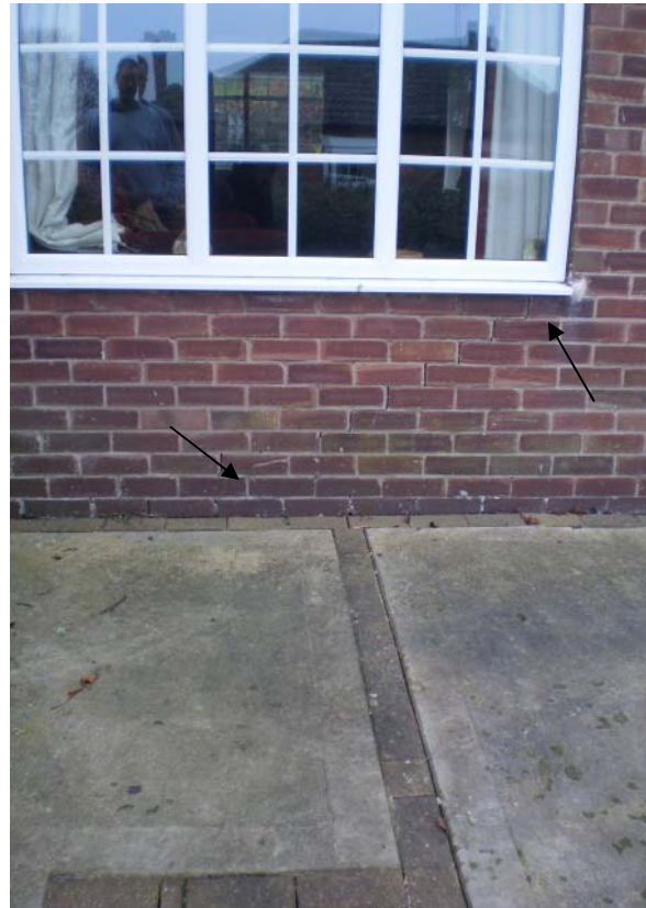
Extension right flank below ground floor window
