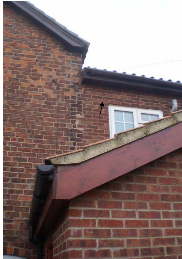
Right hand flank – damage top left of bathroom window
