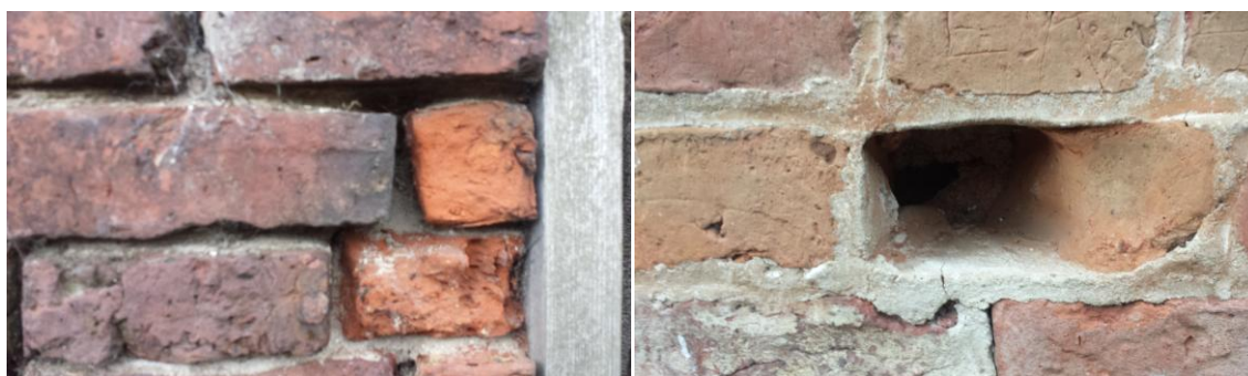
Photograph 6: Representative images showing age related defects in the brickwork.
