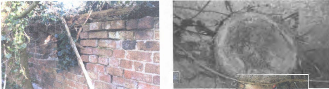
Photograph 8: Ivy and settlement cracks (left) and disused thrush nest (right)
