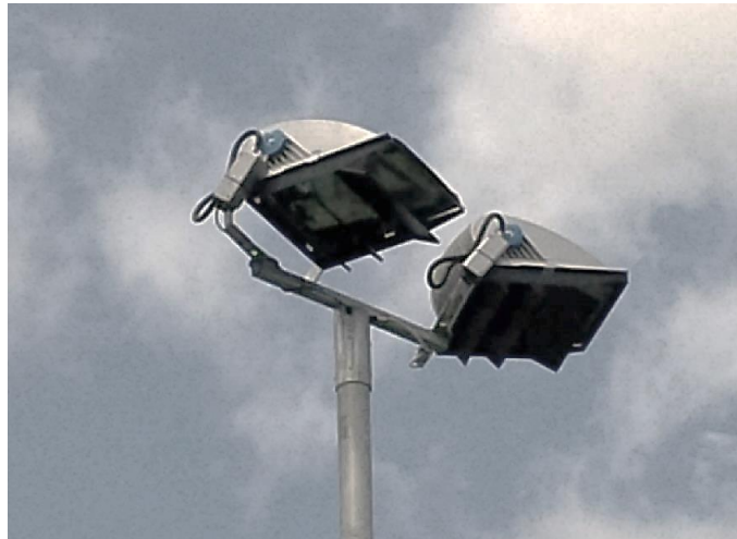
Artificial (Flood) Light Mast c/w Two Luminaires and Optivisors
