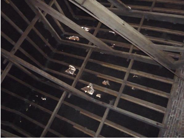
Photograph 5: Gaps in roof (inside barn)
