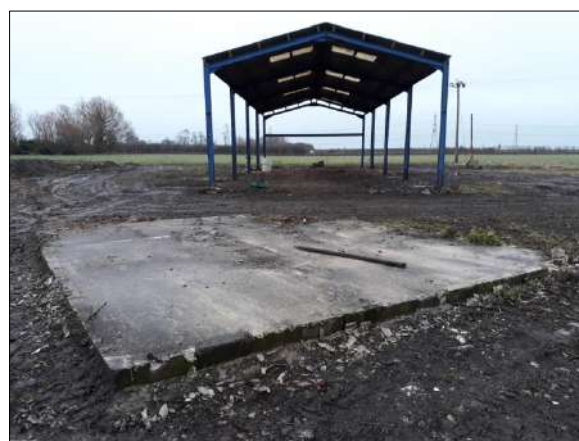
Looking east towards the second steel-framed barn. Note adjacent foundation slab for small building
