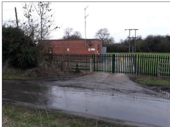
Examples of nearby modern buildings within the EEL landscape: electricity sub-station to immediate southwest of the application site
