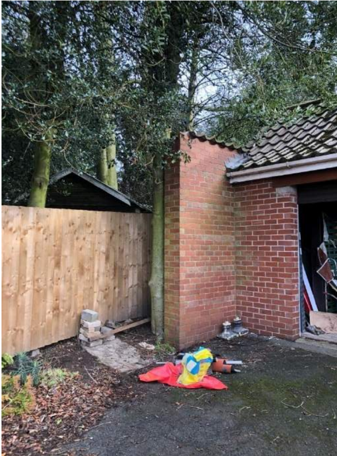
Picture 3 - showing the proximity of holly T4 adjacent to the projection wall of the garage.
