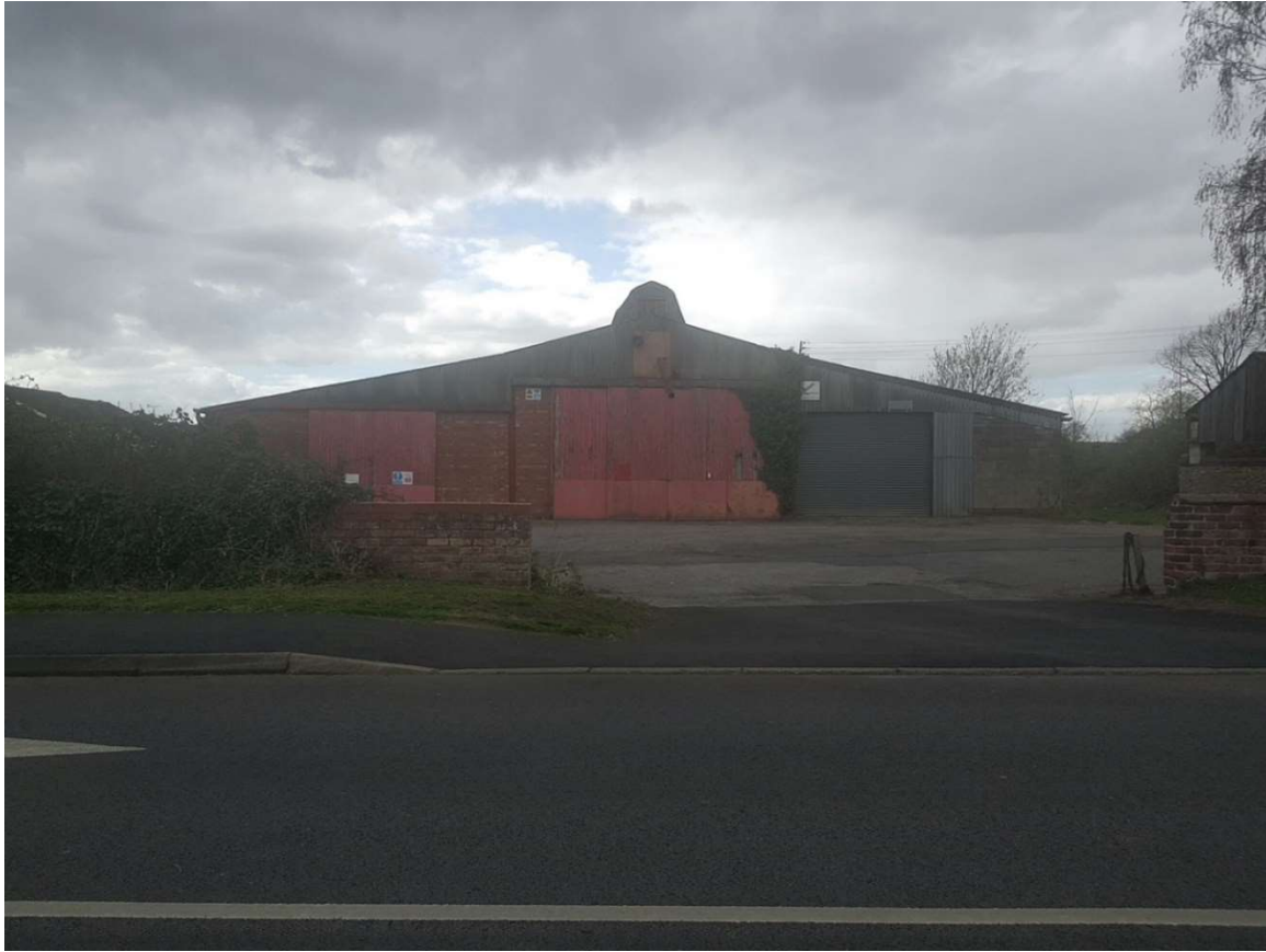
Site entrance into the application site from Scotter Road & view of the derelict barn
