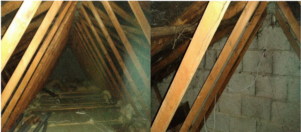
Plate 4.8 – (L) Facing north, the roof void of the extension to the restaurant building. (R) Facing north, the gable end within the roof void of the extension to the restaurant building.
