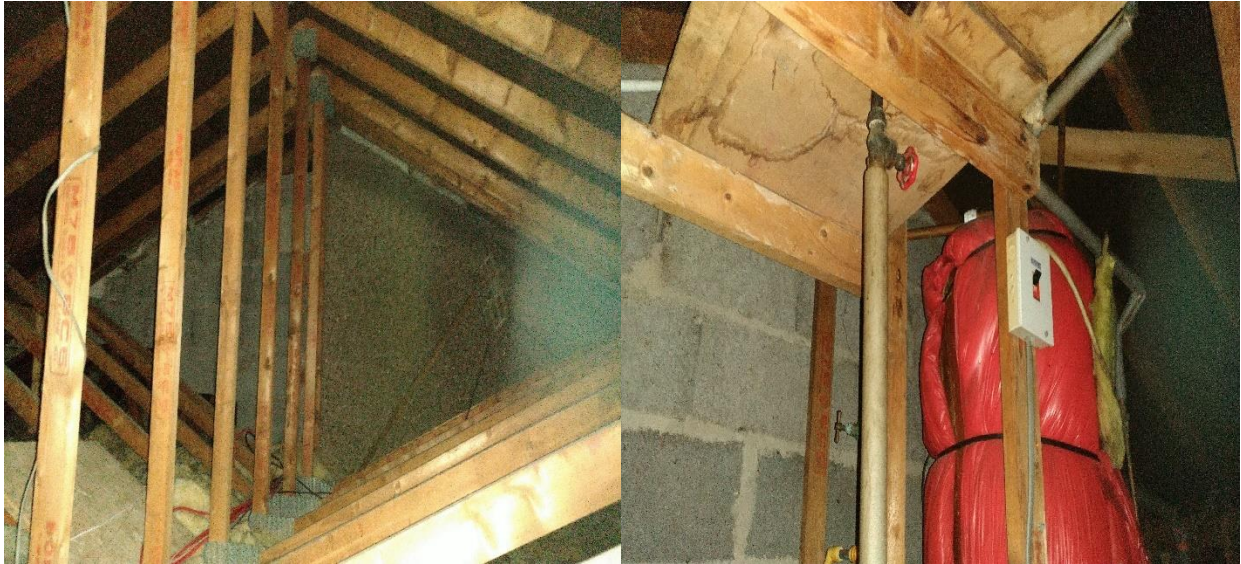
Plate 4.7 – (L) Facing north, the roof void of the single storey restaurant building. (R) Facing south, the gable end within the roof void of the single storey restaurant building.
