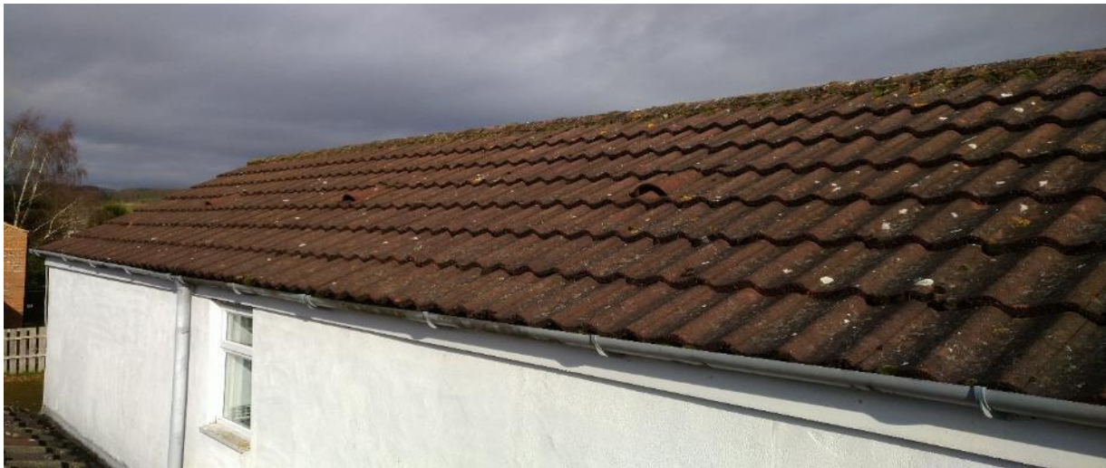
Plate 4.2 - The west elevation
