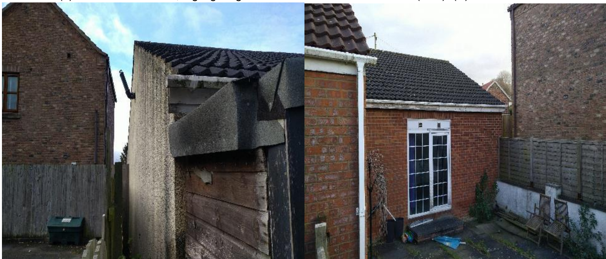
Plate 4.4 - (L) The south elevation (R) – The southern section of the west elevation
