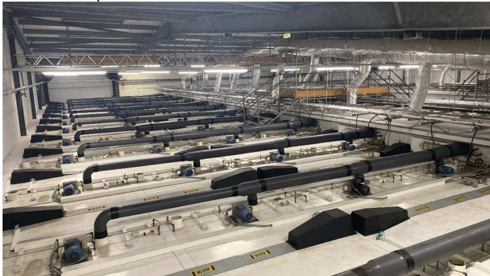
Fans in roofspace above setter corridor
