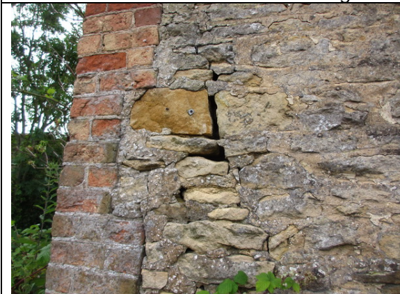
Photo 25: Missing mortar in building 2
