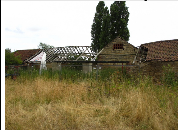
Photo 9: Collapsed building between 6 and 7
