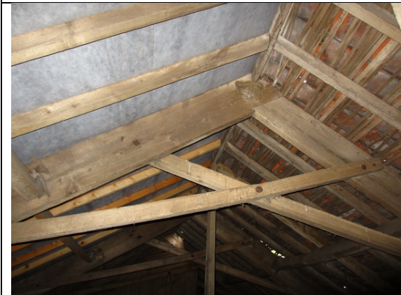
Photo 23: Swallows nest, modern roof membrane and lathes in building 5
