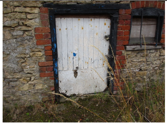
Photo 30: Gaps around door in building 2
