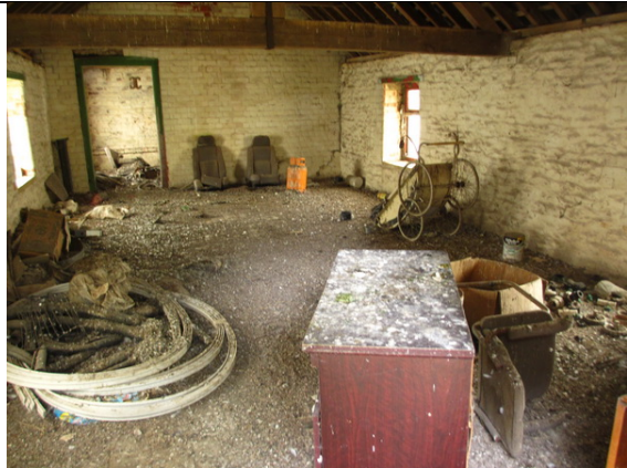
Photo29: Pigeon muck in building 8
