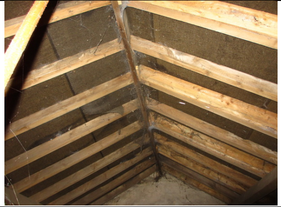
Photo 28: Cobwebs along ridge beam in building 1
