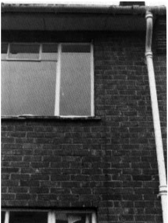
Fig 4 Category 3 damage movements predominantly rotational and horizontal
