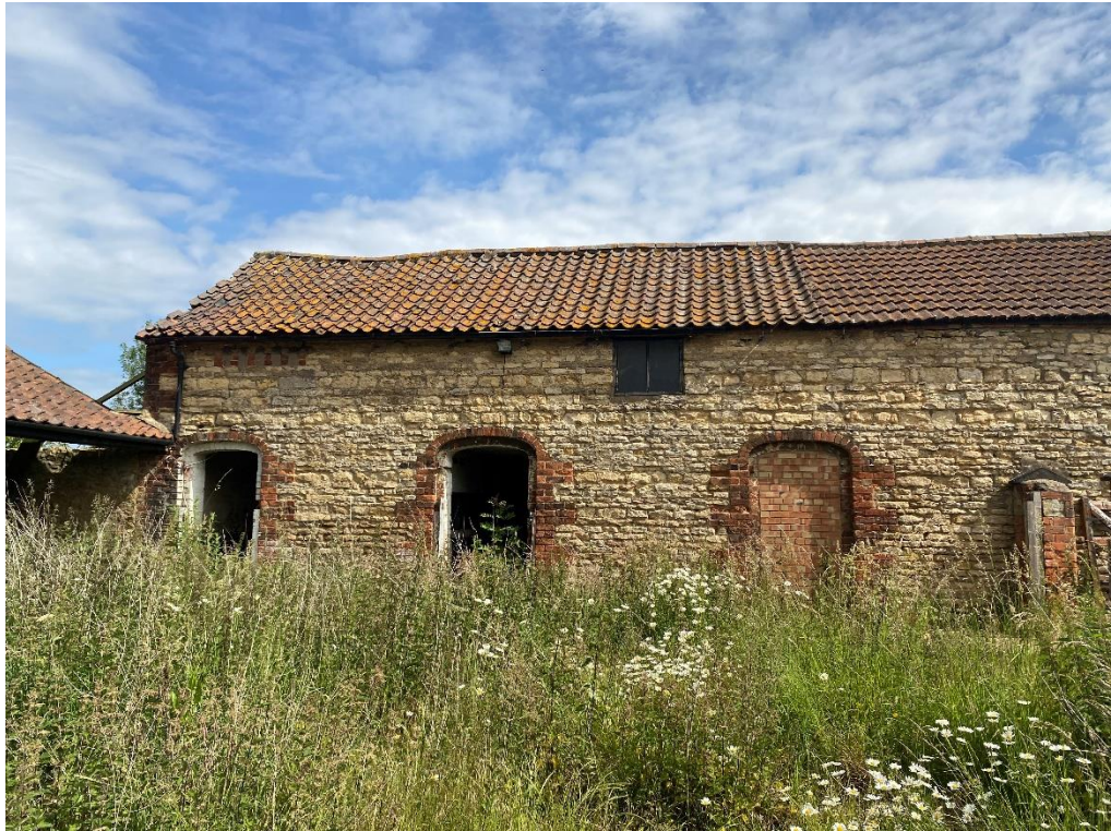
Fig. 27 – Building 3 – south elevation – this is a 2-storey building of stone and brickwork construction under a pantiled covered timber roof with a timber first floor construction
