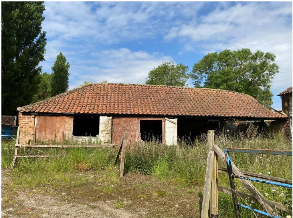
Fig. 20 – Building 1 – east elevation – this building is a mixture of stone, brickwork and modern blockwork wall construction with a hipped pantiled roof on a traditional exposed timber roof construction – partial demolition of this side is recommended within the structural appraisal
