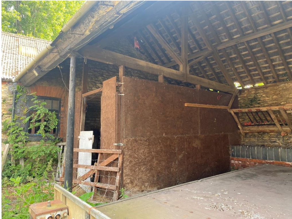
Fig. 43 – Building 5 - the northern bay which is enclosed by timber panels – there is a wooden and brick-built feeding trough along the internal east wall. The roof is supported by King post timber trusses on the lines of the exposed cast iron columns
