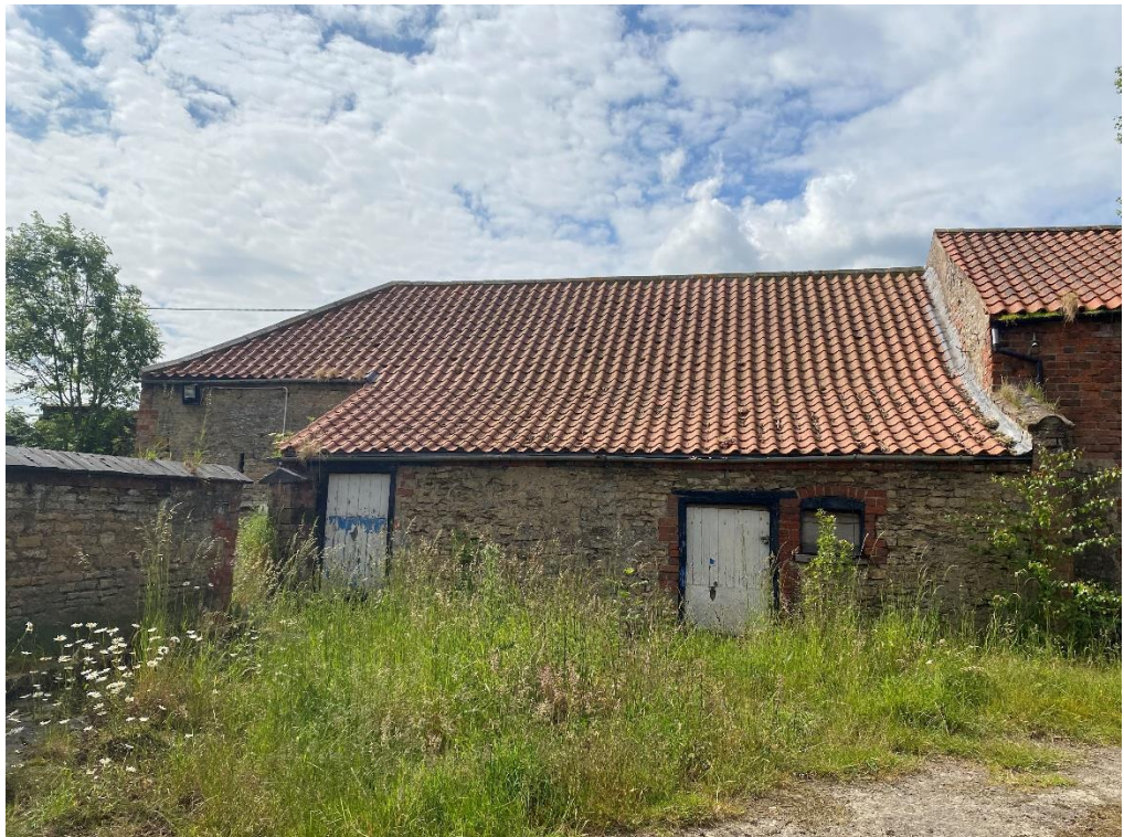
Fig. 44 – Building 6 – western end north elevation – this building comprises one main building of 5-bay construction with two smaller bays housed within the cat-slide roofed extents
