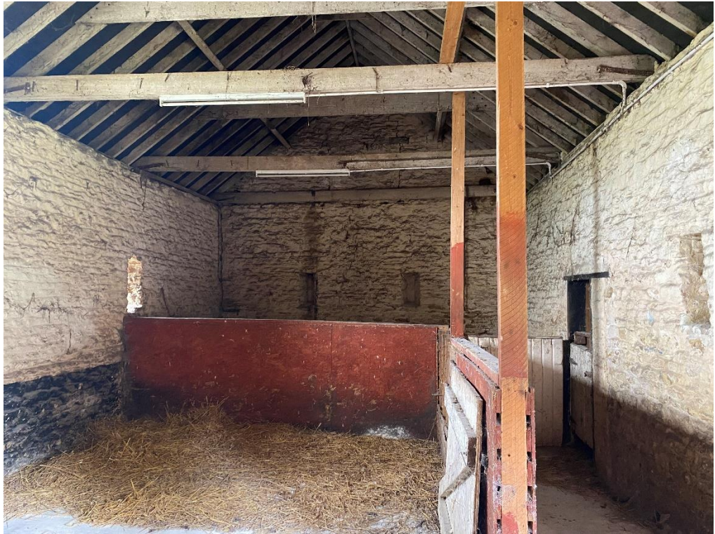
Fig. 47 – Building 6 – the main eastern building which has a timber trussed roof construction with a rough cast concrete floor and stone walls
