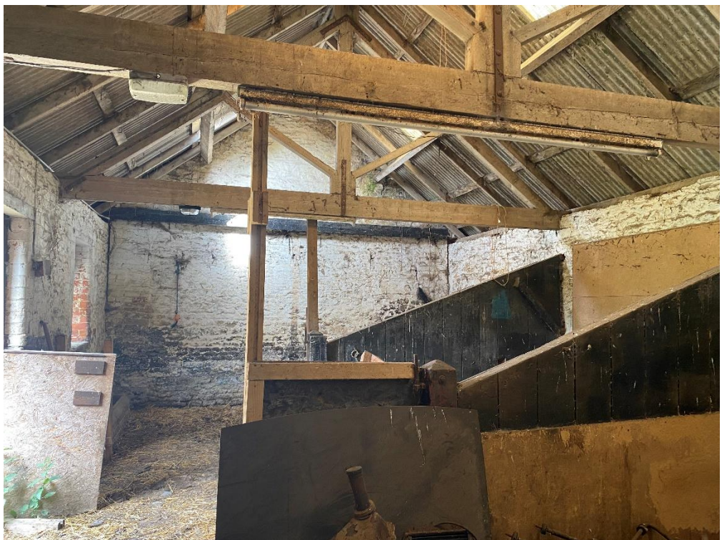
Fig. 36 – Building 4 - the main bay which has a king post timber roof construction and timber stall risers
