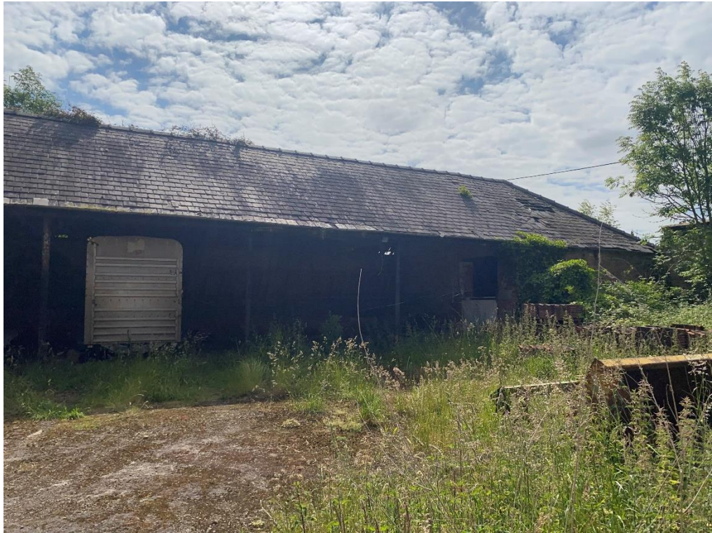
Fig. 37 – Building 5 – west elevation, the northern extents are four open bays with cast iron columns (the fifth northern bay is enclosed with a timber panel wall) – the southern end is a single enclosed bay with stone walls
