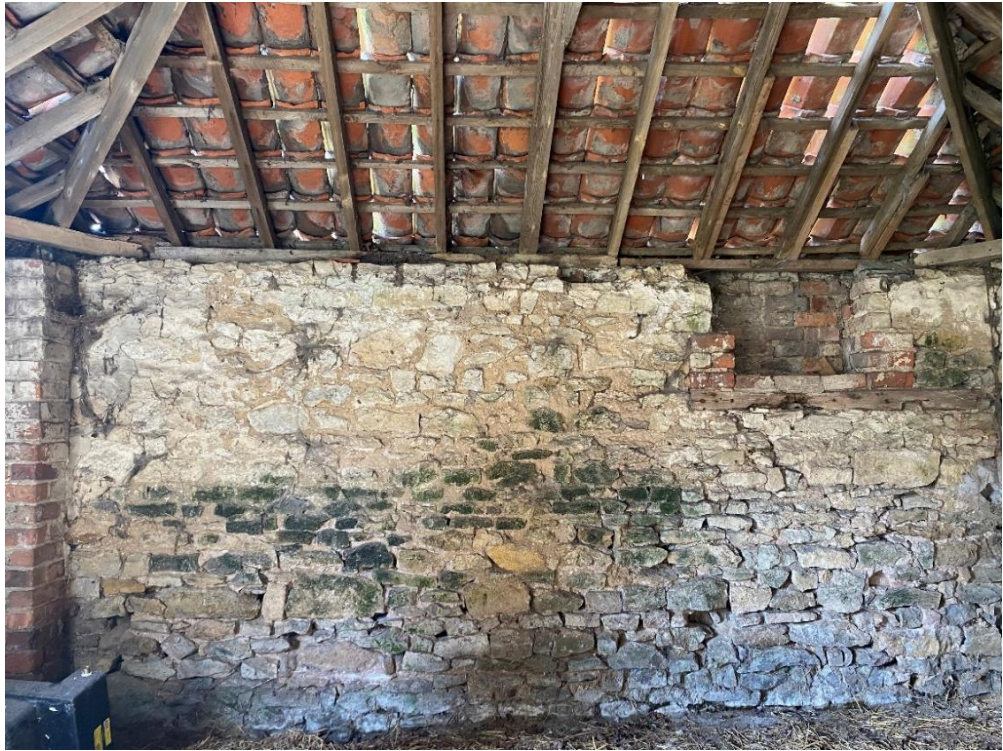
Fig. 21 – Building 1 - the internal southern end – the floor to this building is partially concrete construction
