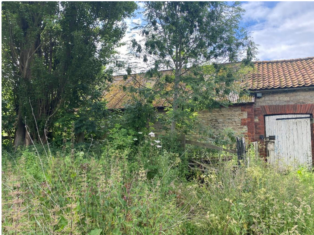
Fig. 34 – Building 4 - much of the north elevation is obscured by vegetation
