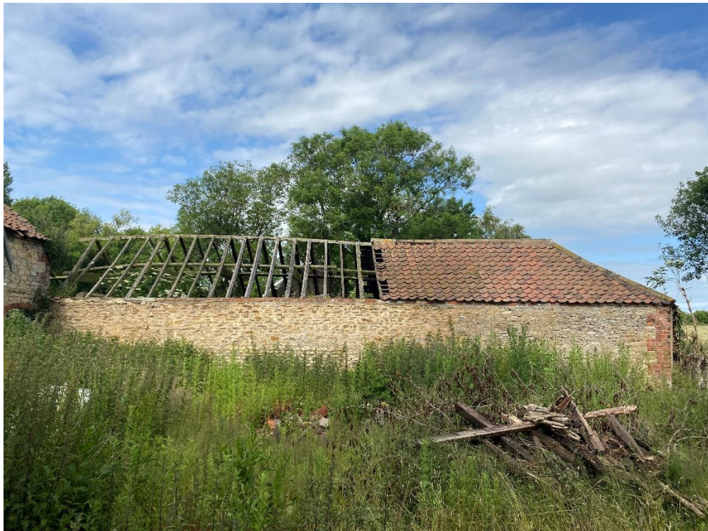
Fig. 26 – Building 2 – eastern elevation – careful demolition and rebuilding of this structure is recommended in the structural appraisal
