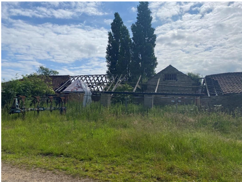
Fig. 24 – Building 2 – west elevation – this building may have been subject to a previous fire – large parts of the roof covering are missing, roof timbers are deformed and there is vegetation growth affecting the built fabric
