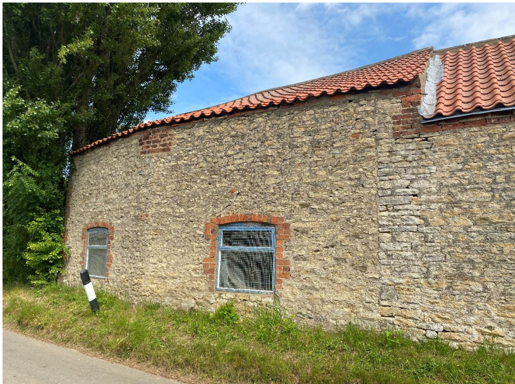
Fig. 50 – Building 6 - the south elevation of the western element – internal access to this building was not possible
