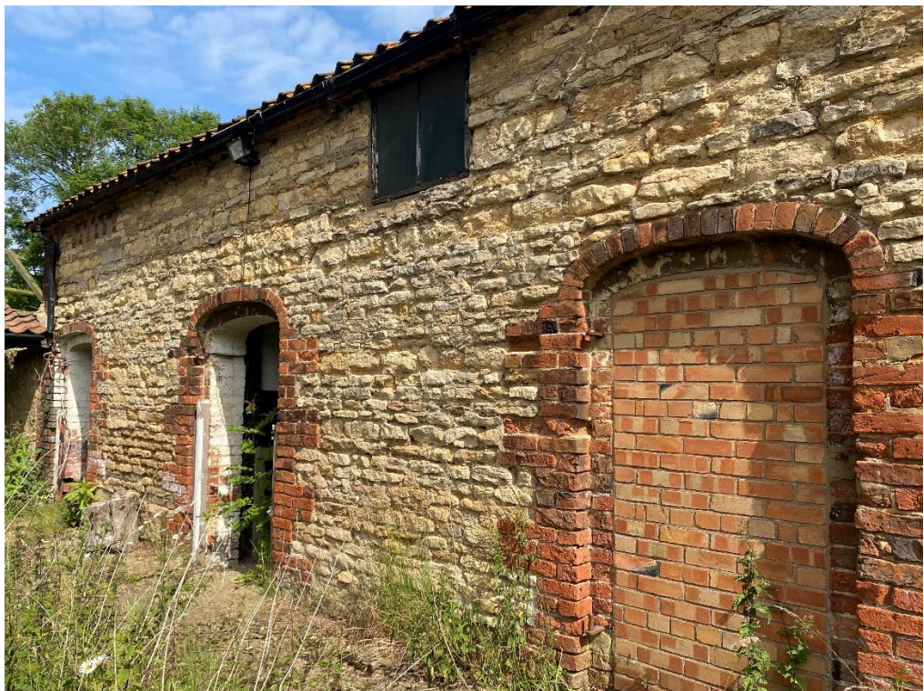
Fig. 28 – Building 3 - part of the south elevation with the arched door openings onto the main enclosed yard and showing a blocked door opening and a boarded first floor window
