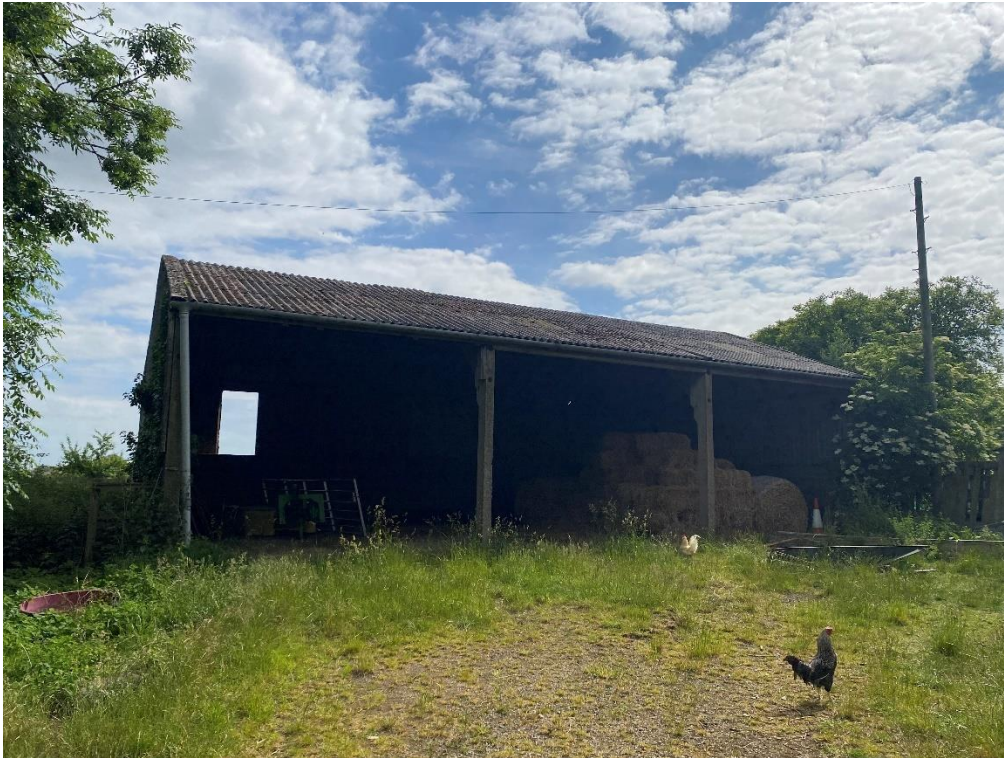
Fig. 57 – Building 8 – the south side of this open shed, which has a prefabricated concrete framed construction – this building does not form part of the application development proposals
