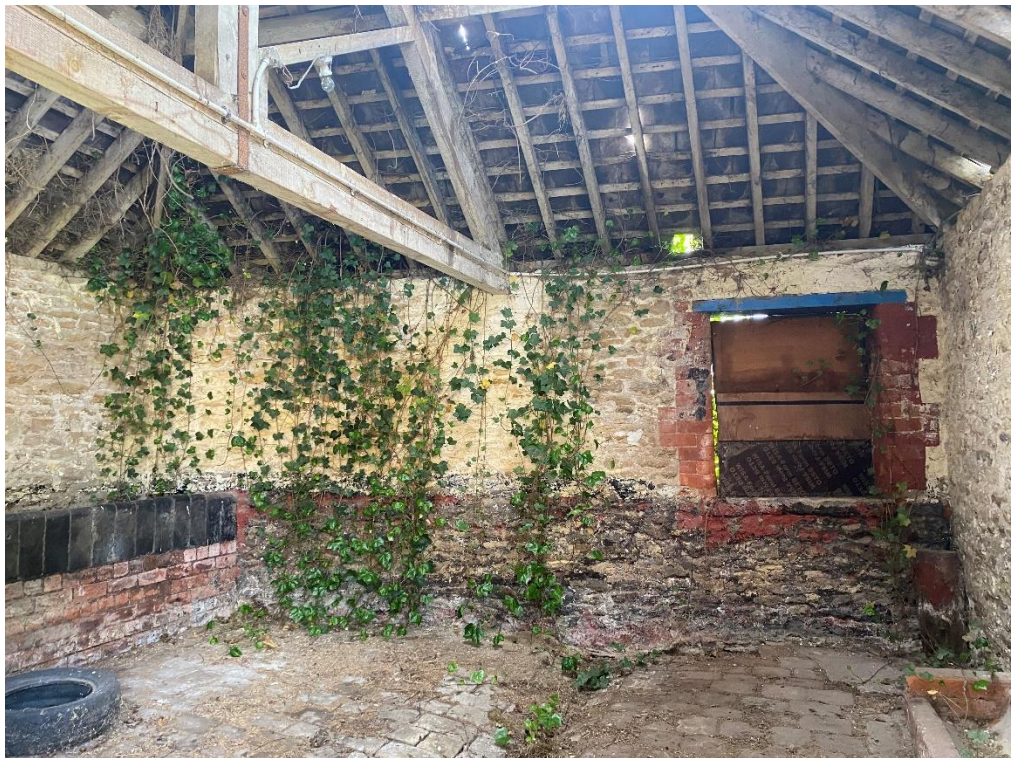
Fig. 40 – Building 5 - the southern bay has a boarded up window opening on its south elevation. The floor has a dished profiled cobbled floor. The roof has a hipped king post roof construction. There is a brick built feeding trough to the internal west side.
