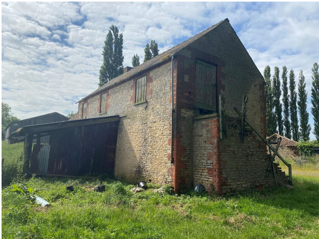
Fig. 52 – Building 7 – showing the west and north sides – there is an open lean-to timber construction to the north side and an external stair to the west side
