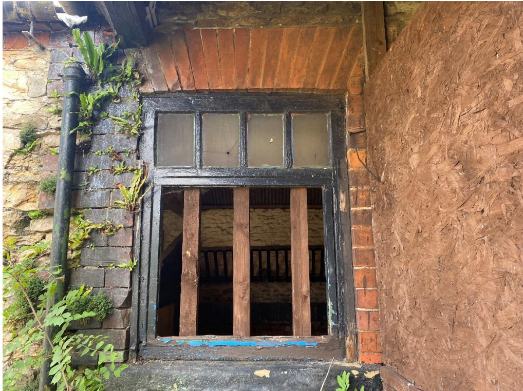
Fig. 33 – Building 4 - a timber window to the south elevation, which sits under the roof overhang of the adjoining building 5.
