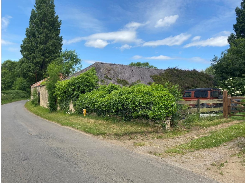
Fig. 39 – Building 5 – the southern end which sits tight to North Street – the roof has a hipped end with a natural slate roof covering
