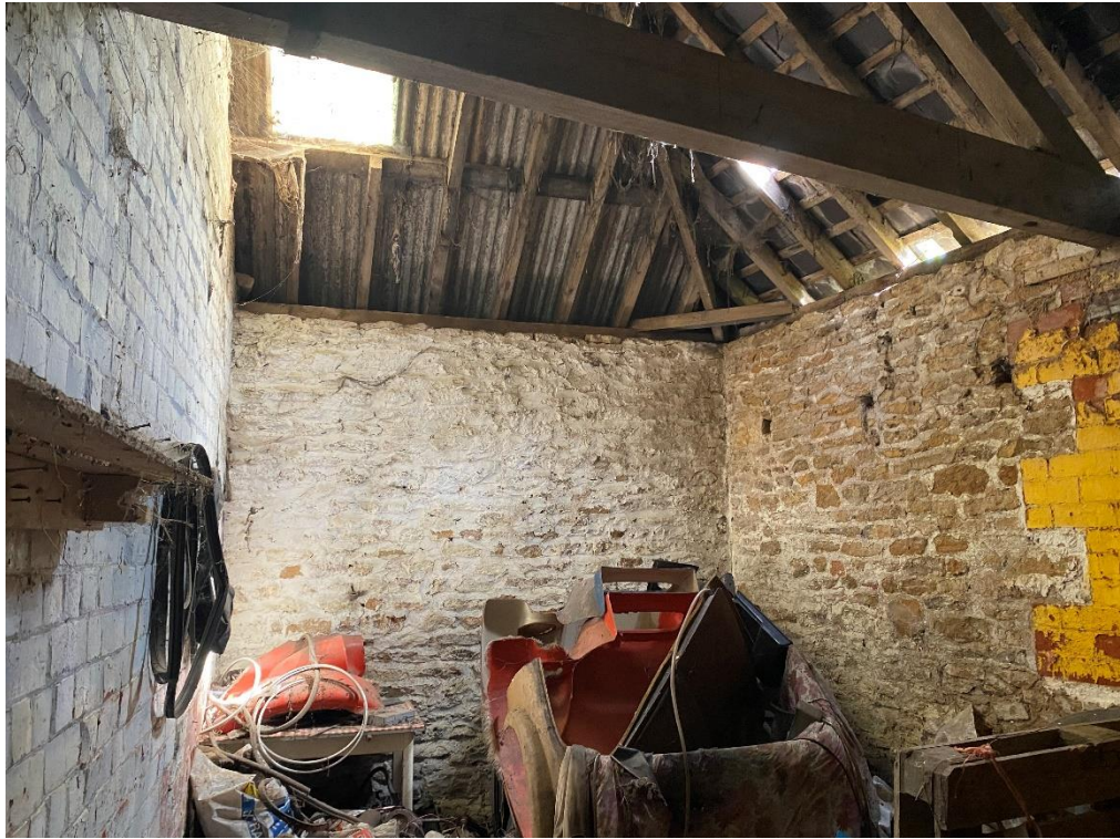
Fig. 35 – Building 4 – part of the eastern end bay – this building comprises a larger main bay accessed to the south off the main yard with an internal door to the end bay shown above
