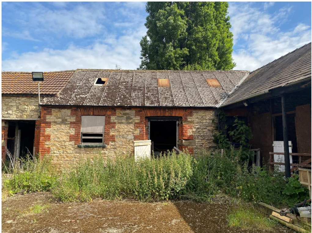
Fig. 32 – Building 4 – south elevation showing the profiled sheet roof covering, rooflights and brick detailing to the door and window openings
