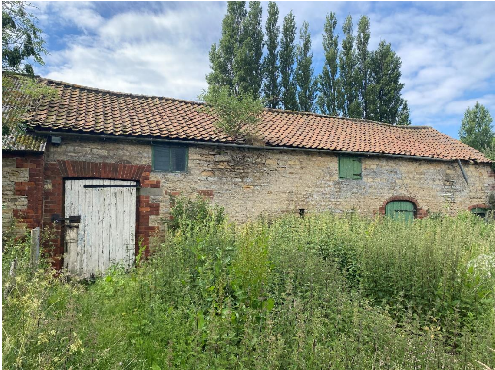
Fig. 29 – Building 3 – north elevation, which has a substantial timber boarded door opening and an arched headed door opening and ground floor windows opening to the western end
