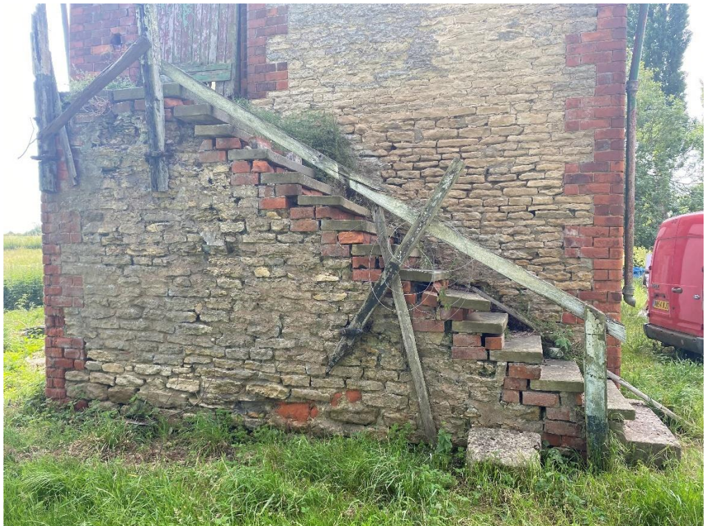
Fig. 54 – Building 7 - the external stair, which is recommended for demolition due to its structural instability
