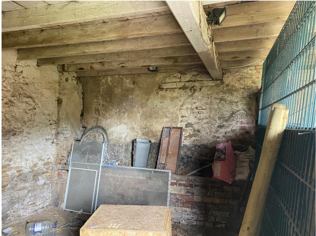
Fig. 31 – Building 3 - renewal of the first-floor construction is recommended in the structural appraisal – this building is sub-divided into 3 bays with a further timber division shown in fig. 30 above – there is a brick-built feeding trough in the easterly bay
