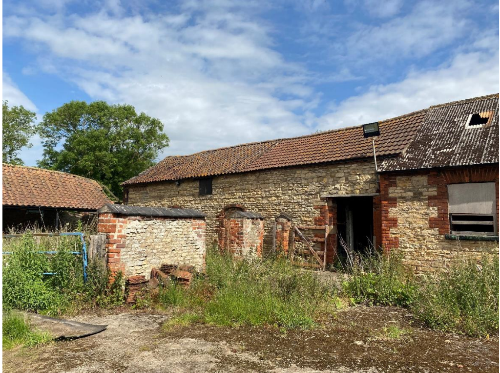
Fig. 14 – part of the northern range of the main yard – the yard is divided by some freestanding stone and brick-built walls
