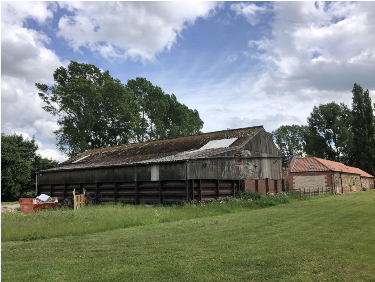
Image 3 – Existing barn viewed from the North West. This also shows a traditional stone barn, which has been converted in recent years.
