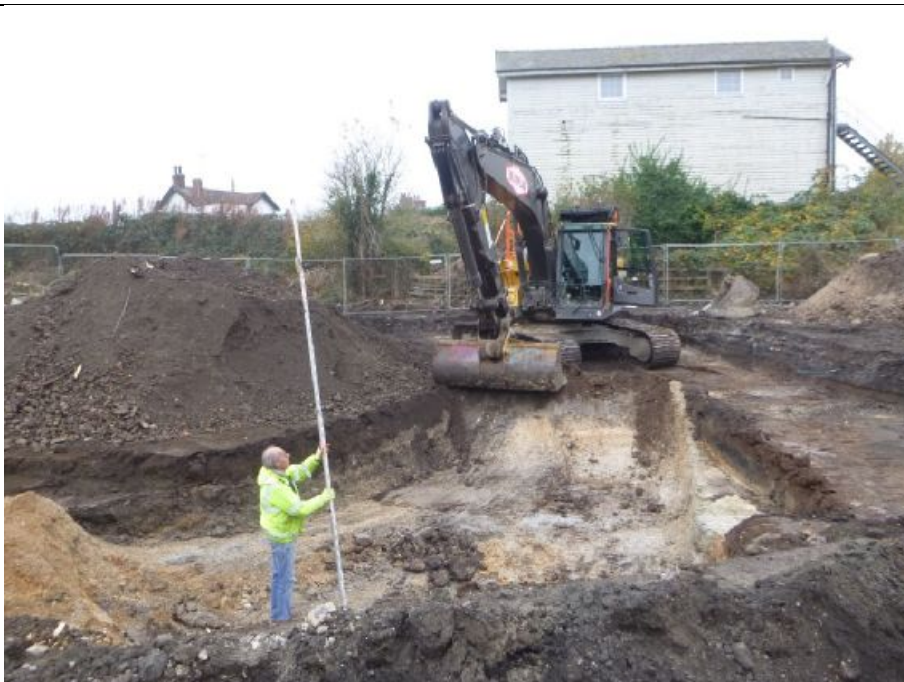
Site photo: 4 Date: 16 October 2021 Photo direction: Northwest Description: The north part of the completed remediation excavation
