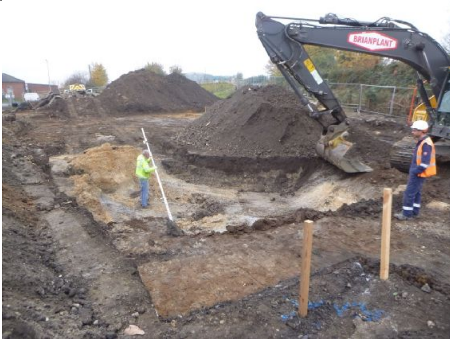
Site photo: 3 Date: 16 October 2021 Photo direction: West Description: the completed remediation excavation
