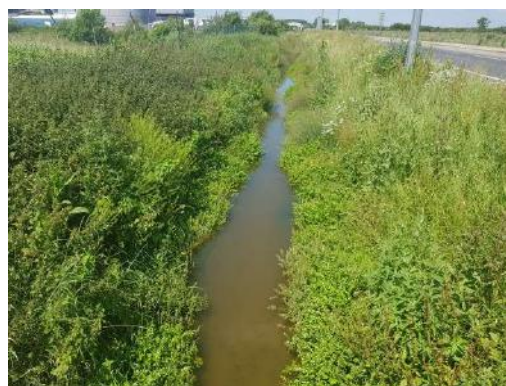
Photograph 13. The drain parallel with western carriageway of Rosper Road from the IDB outfall looking north.
