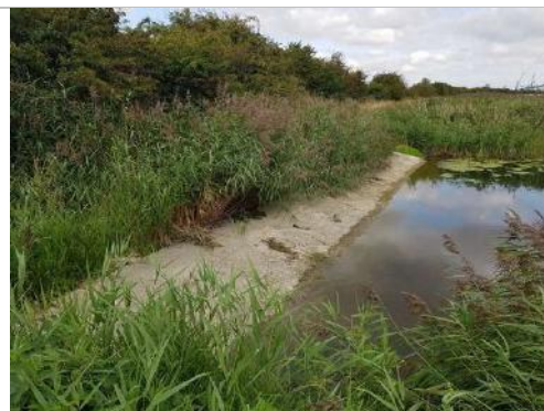
Photograph 16. IDB drain as it trips over the spillway into Rosper Road pools.
