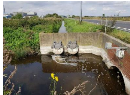
Photograph 12. The drain along Rosper Road connects to the IDB drain via a flap valve. The IDB drain then runs eastwards under Rosper Road via an open culvert.
