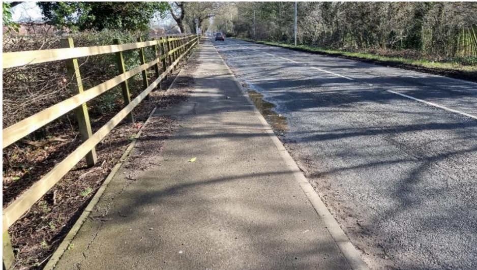
Photo 2: Footway on Burringham Road
