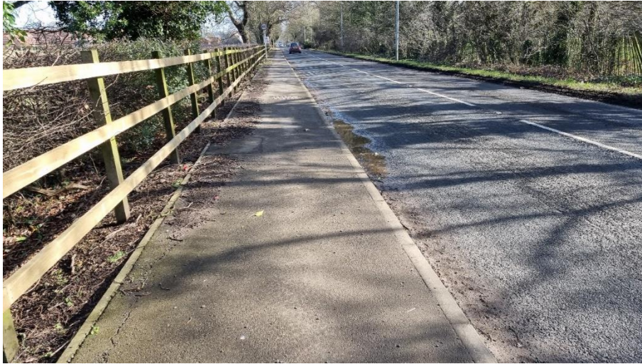
Photo 1: Footway on Burringham Road
