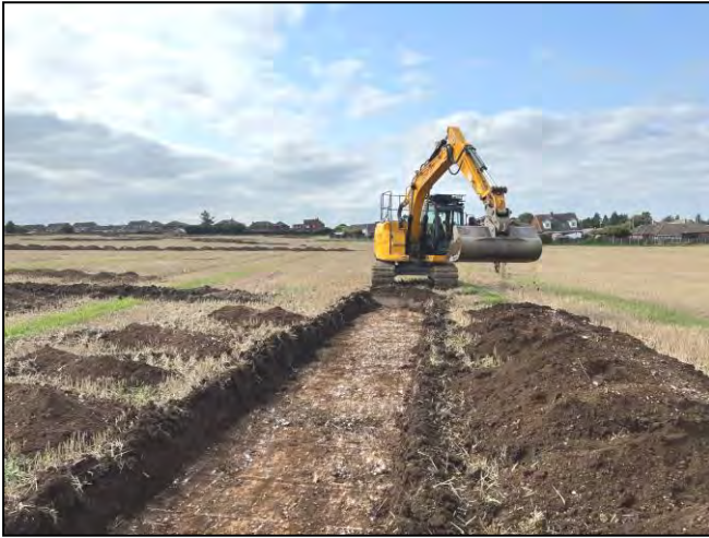
Plate 3: Working shot during machine excavation of Trench 10, looking west towards the recent housing development on Glebe Way.
