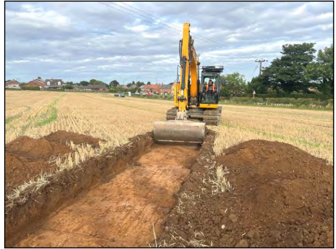
Plate 4: Working shot during machine excavation of Trench 4, looking west along the edge of the field bordering Barrow Road.
