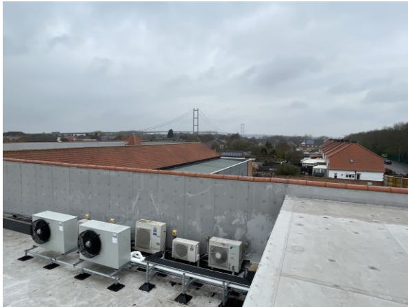
View of Mechanical Equipment on Roof
