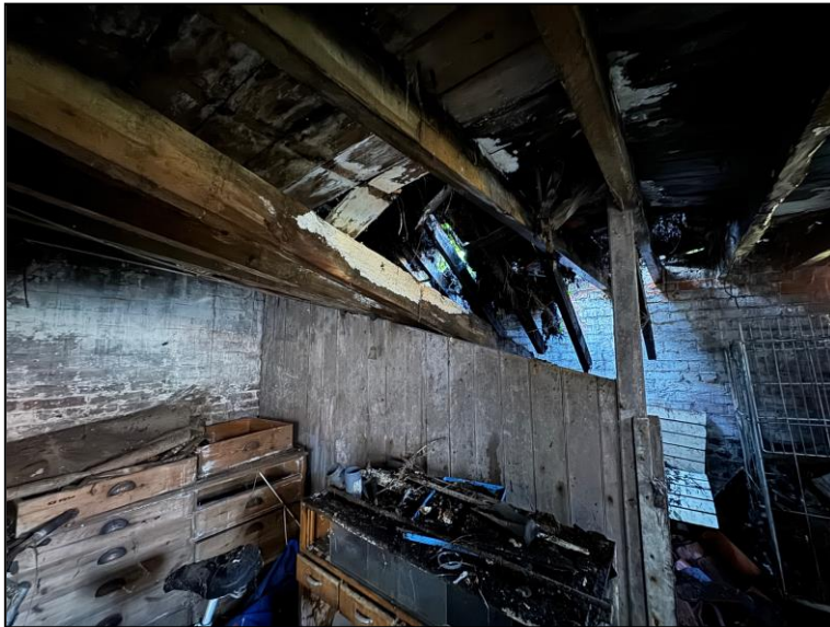
Photo 7 – hole/damage to single storey roof
