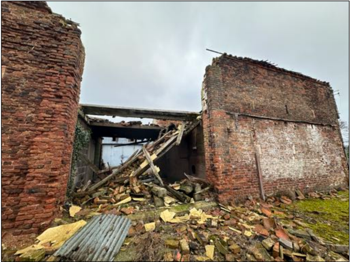
Example of debris from collapsed roof
