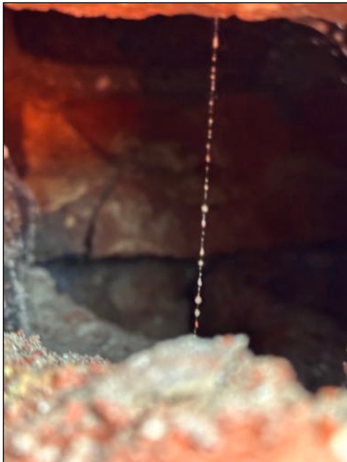
Example of cavity within wall which would provide low habitat potential
