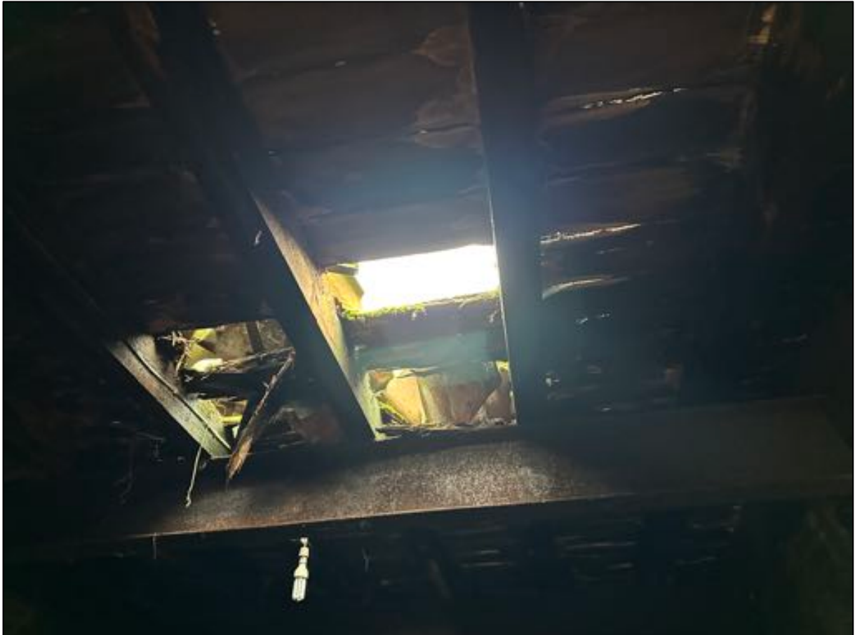
Example of upper flooring beginning to collapse due to exposure to the elements
