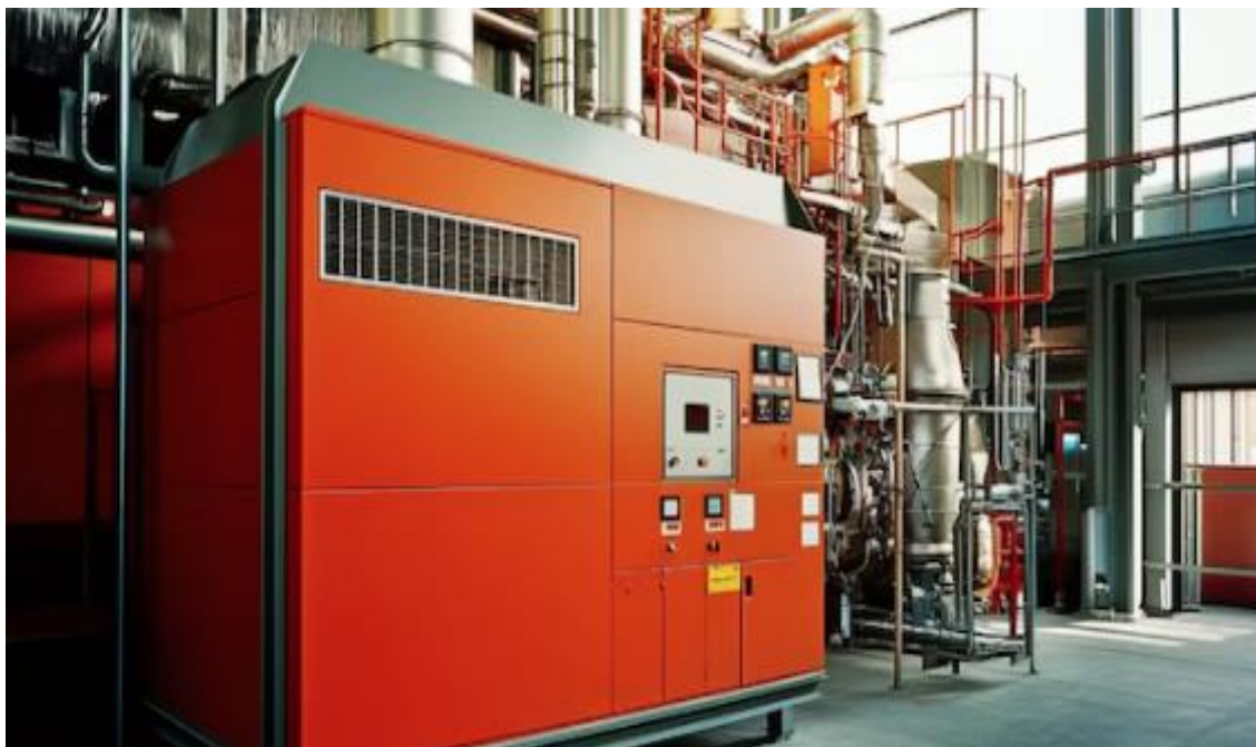
Figure 3.3: Combined Heat and Power (CHP) Plant
