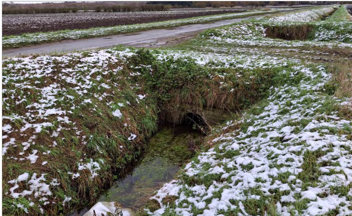
Plate 9: View of drainage dyke parallel to Brumby Common Lane with stone culverted field access
