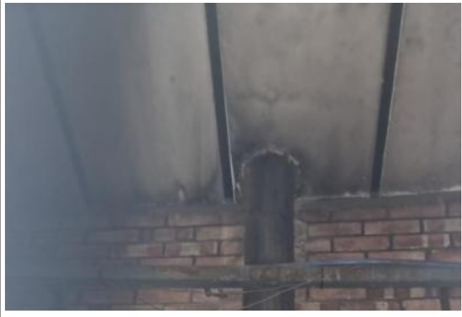
Mental flue pipe in area 2
