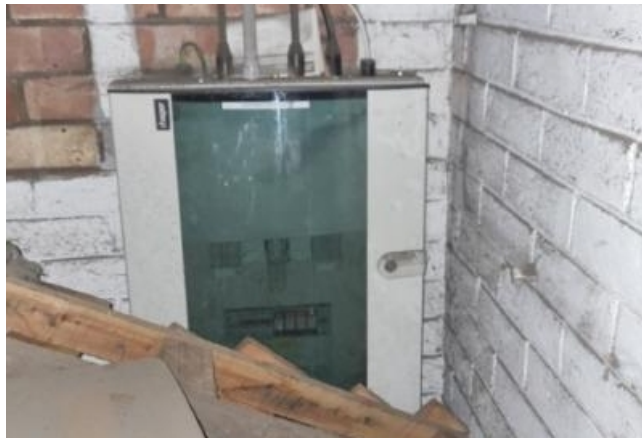
Modern Fuse Box in area 2
