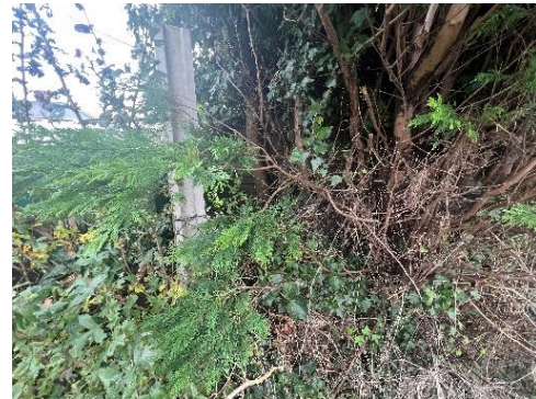
Figure: 10 Further evidence of insecure site boundary line– H&S risk
