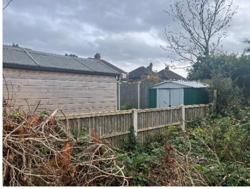
Figure: 7 Low level fencing providing limited security from intruders – H&S risk
