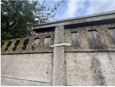
Figure: 13 Unsecure and unstable concrete panel fencing – H&S risk
