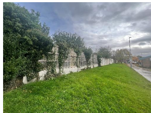
Figure: 12 General view of unsecured east boundary – H&S risk
