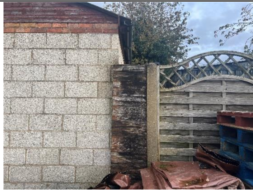
Figure: 3 Previous patch repair to site boundary
