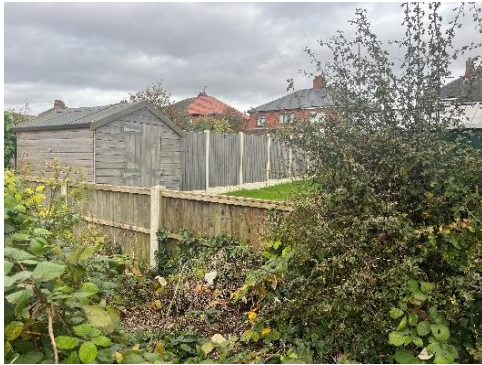
Figure: 9 Evidence of insecure site boundary line – H&S risk
