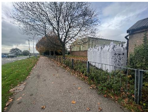
Figure: 17 Inadequate security fencing to site boundary leaves school at risk of intruders entering the site unknowingly – H&S risk
