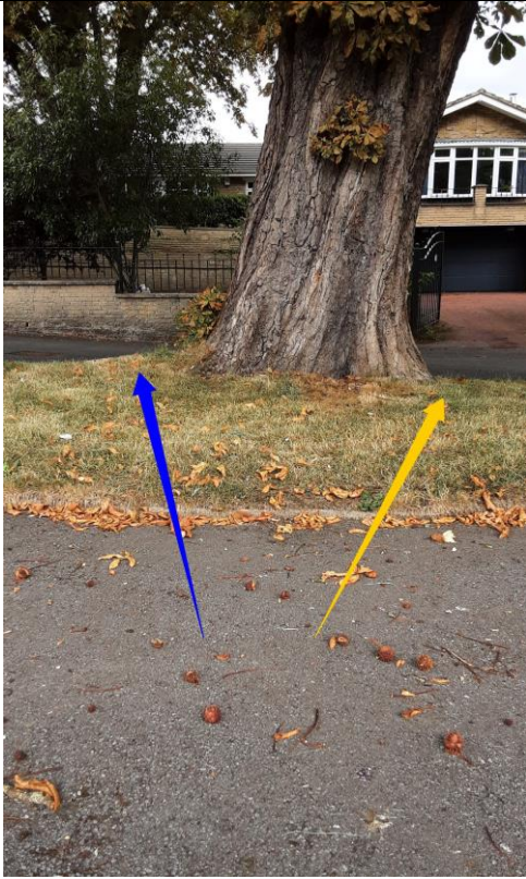
Root heave shown by the blue arrow west, and sunken ground yellow arrow east.
