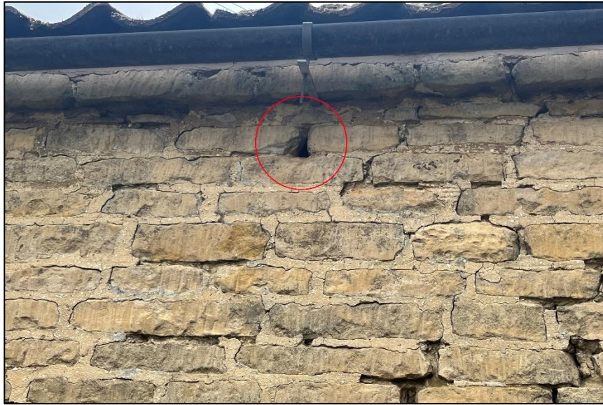
Photograph 3: A potential roost feature within the stonework on the northern elevation of the property (circled in red)
