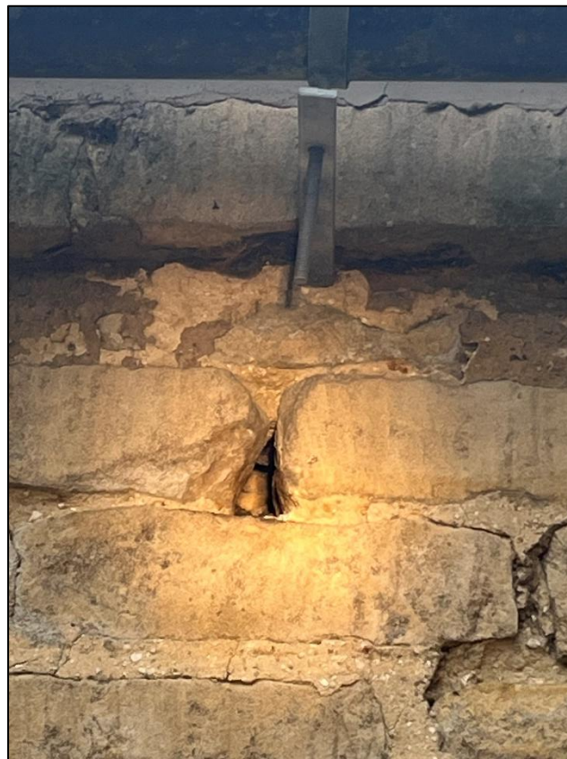
Photograph 4: A potential roost feature within the stonework on the northern elevation of the property (close up)
