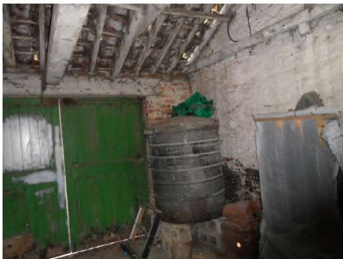
Plate 19 Dampness within the timber floor members in the smaller ground floor Garage area.
