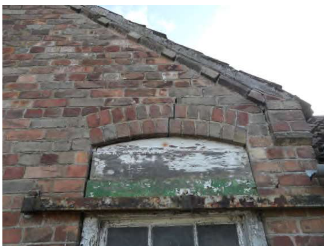
Plate 5 Cracking above the right hand window (Room 3).
