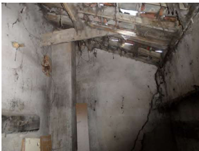
Plate 15 Compromised roof within Room 1.
