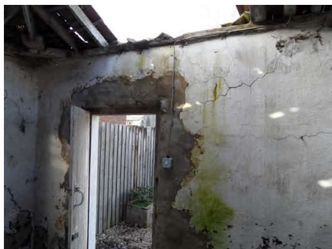
Plate 18 Missing section of roof and perished plaster walls within Room 2.
