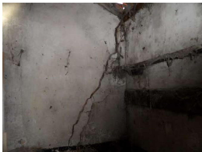
Plate 16 Rotational cracking on the eastern wall within Room 1.
