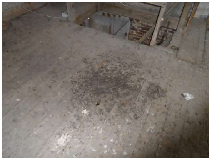
Plate 25 Damaged floor timbers (seemingly associated with bird droppings).
