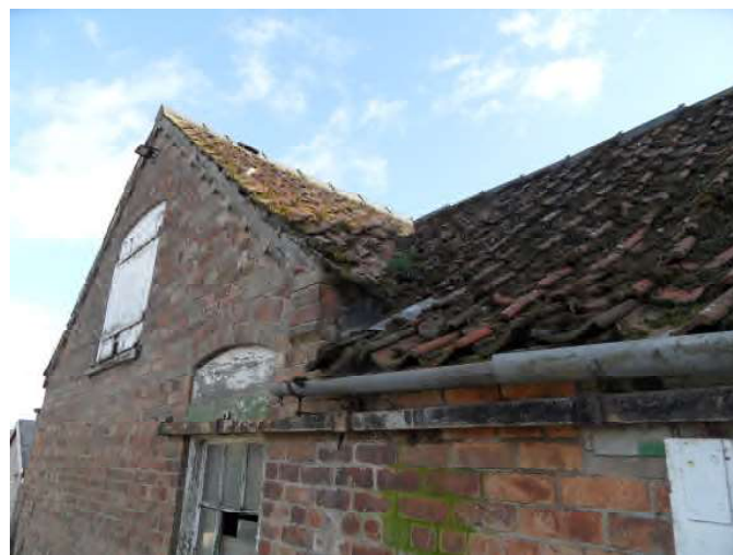
Plate 4 Uneven roof tiling around valley between the Stable and Room 3.
