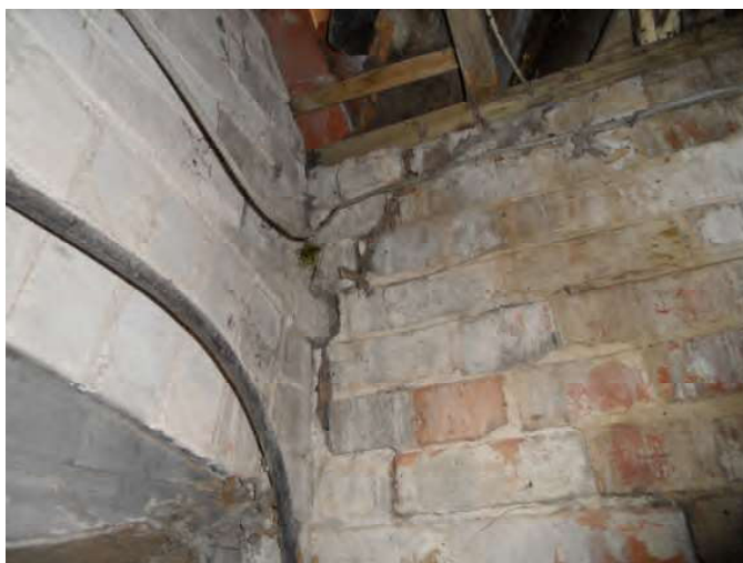
Plate 29 Cracking at high level in the south western corner of Room 3.
