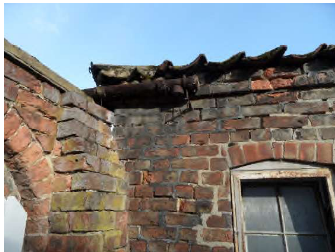
Plate 14 Cracking over west elevation window opening.
