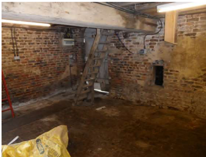
Plate 21 North eastern corner of the Main Barn (dampness noted in principal timber adjacent to the pattach plate strap).
