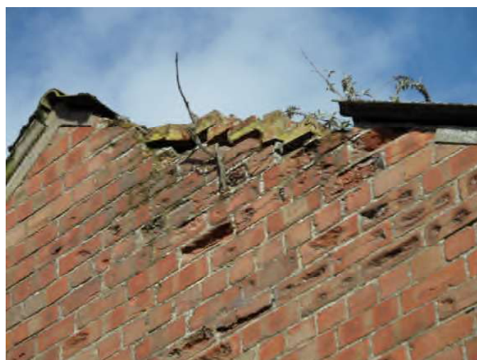
Plate 12 Damaged brickwork on the south western roof slope interface on the Main Barn.
