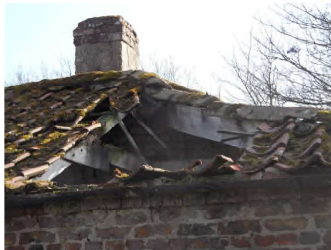
Plate 2 Collapsed roof over Room 2.
