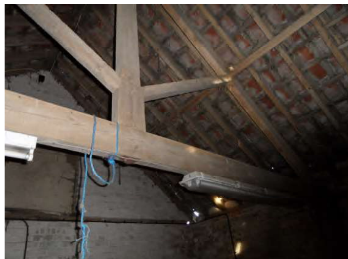
Plate 30 Principal Roof truss in Room 3. Daylight visible sporadically within roof tiling.
