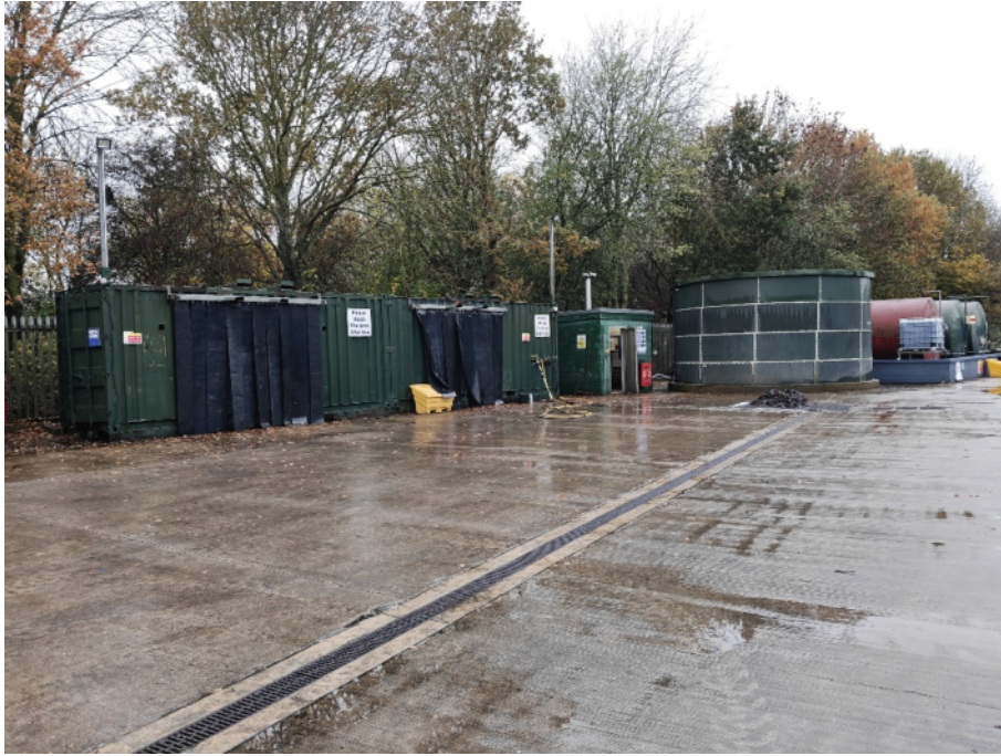
Site walkover photo: 26 Date: 11 Nov 2025 Photo direction: East Description: off-site wash down area, pump house and tanks
