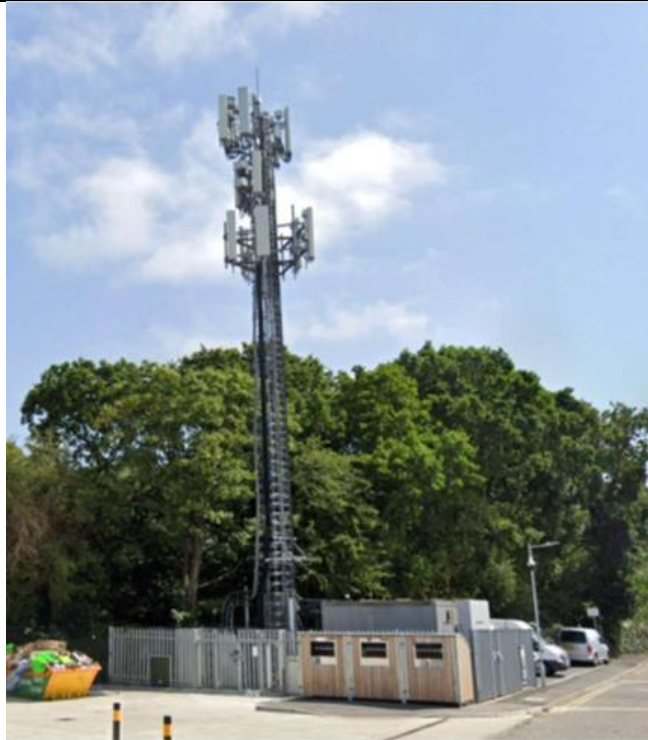
Image 2a: Example of a lattice tower with associated compound
