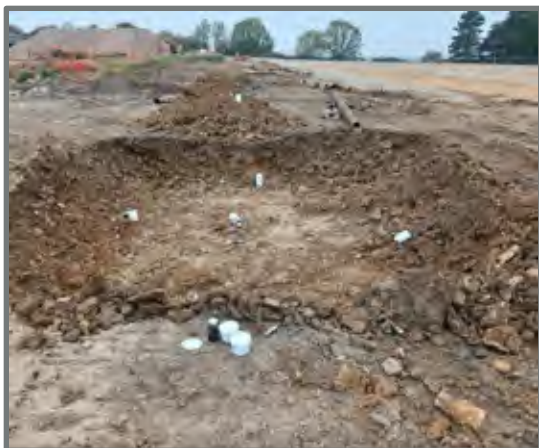
Figure 11. Clean base and sides of hotspot TP9
