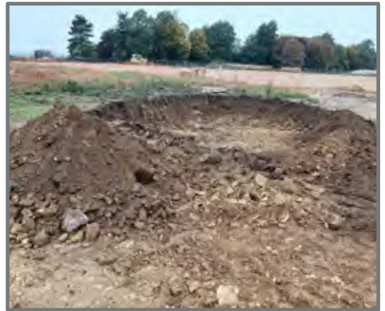
Figure 10. Clean base and sides of hotspot TP37
