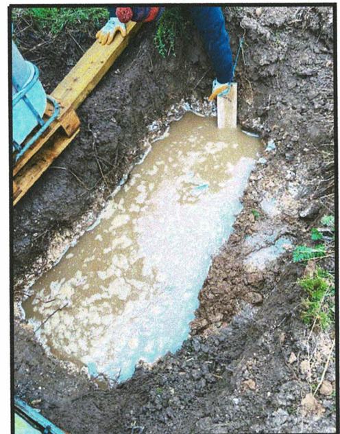
Water fill prior to timing from 75%
