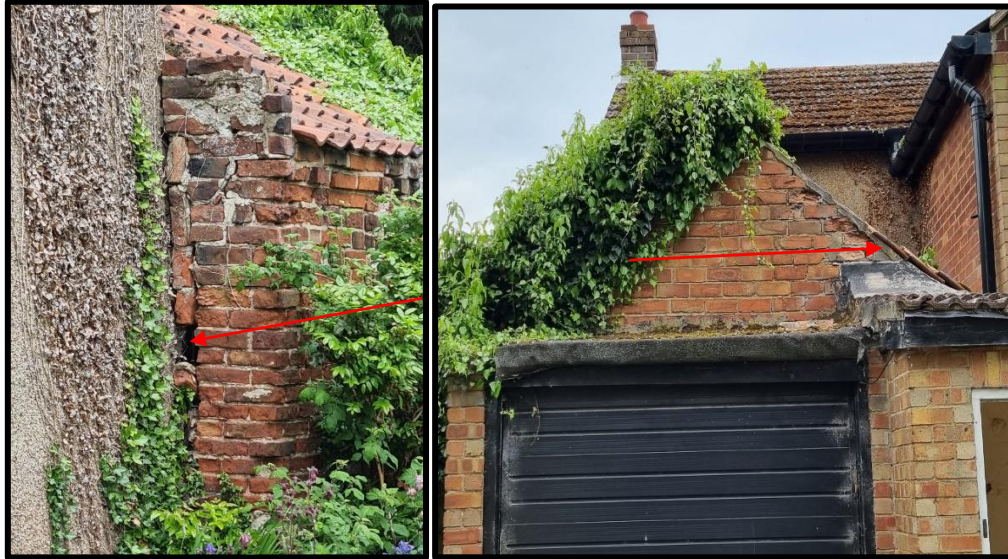
Figure 4: Fissures within the garage.
