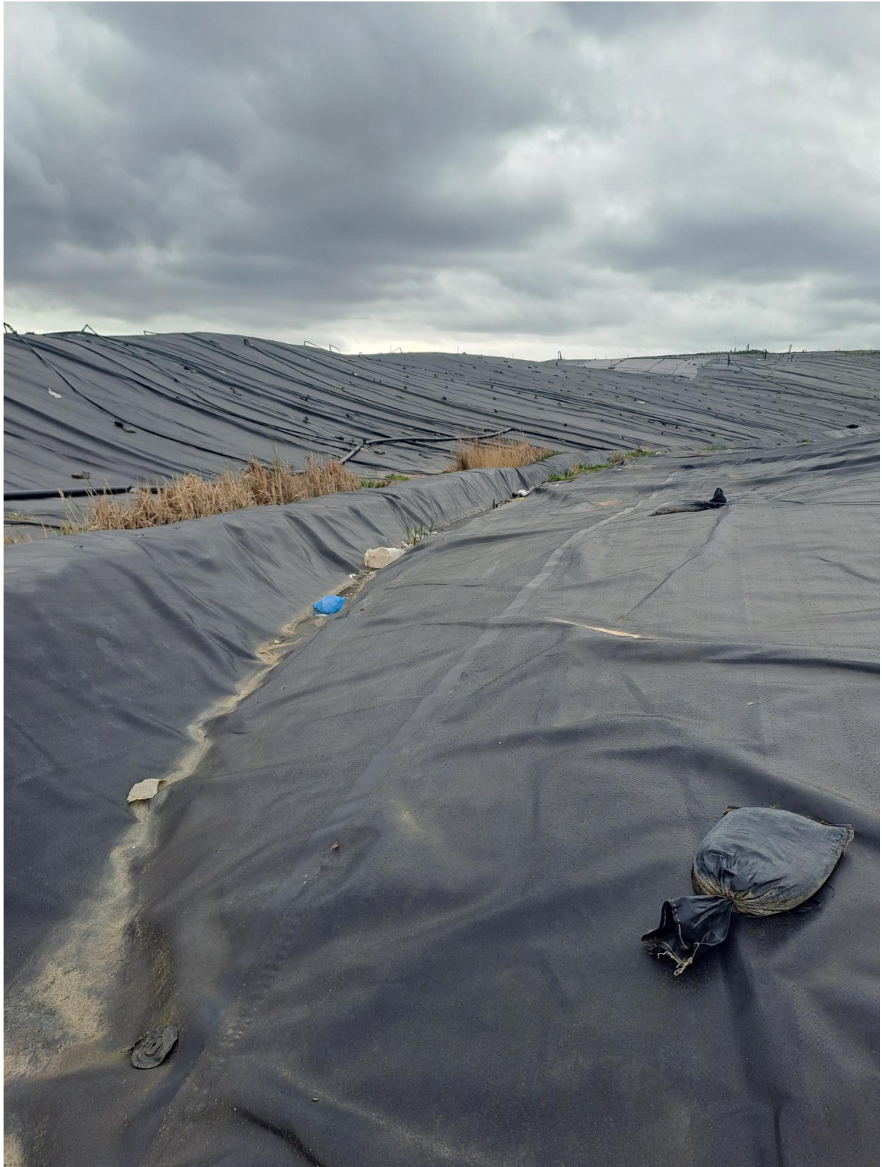
Photo 7: Large valley through Area 1. Taken from the north of the site, looking south
